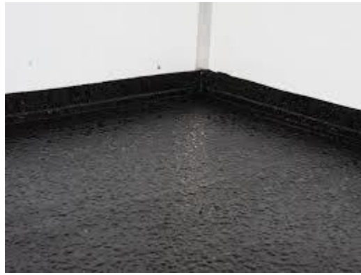
Figure u: Rubberised floor
